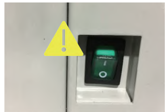
▲ Compressor Switch (i.e. “Cool Switch”)
